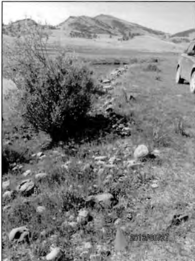
Figure E-1. Bank stabilization above the ordinary high water mark (OHWM) of Sheep Creek at BW-1. Material to remain.
